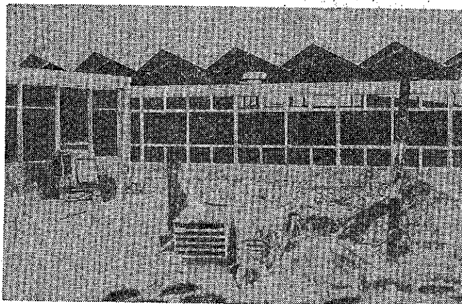
Construction of the new wing progresses as shown by recently erected gables.
